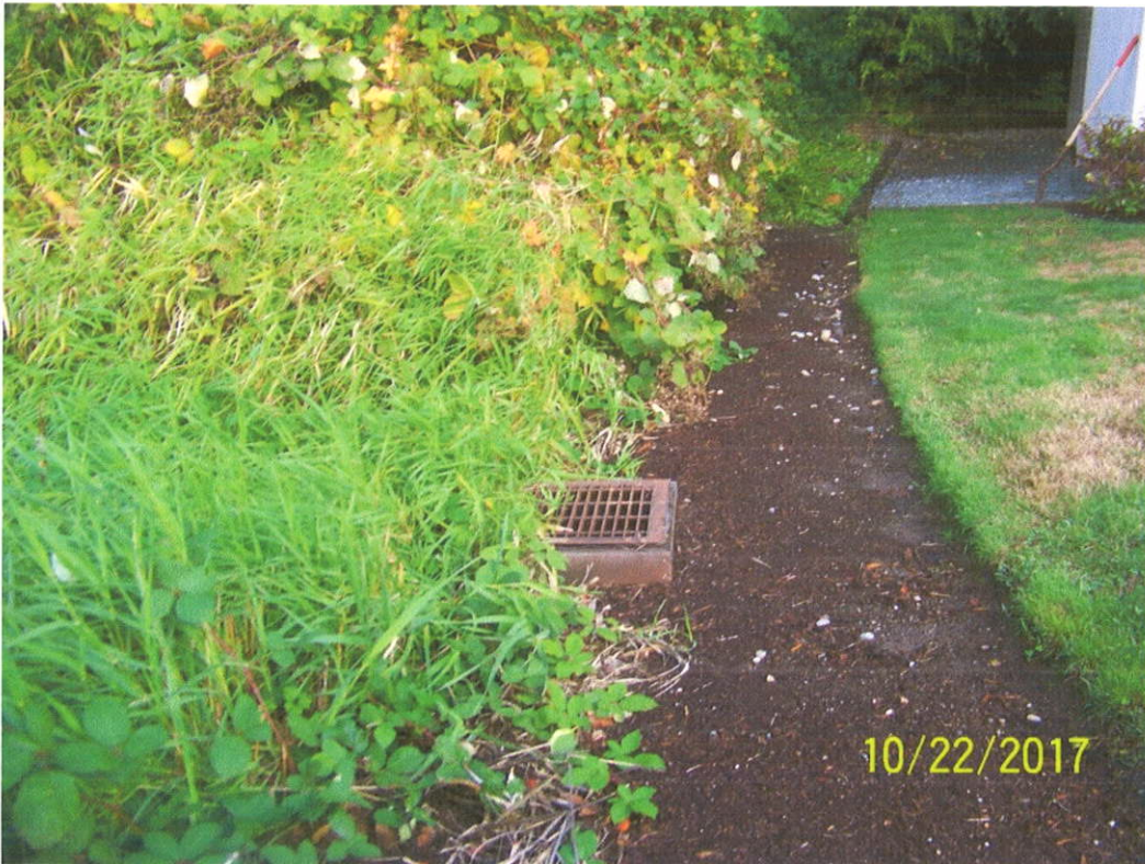
3) Storm drain on eastern Property boundary, intercepting stormwater from residence to the east.
